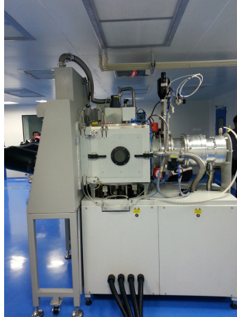
View from side showing coater service door
