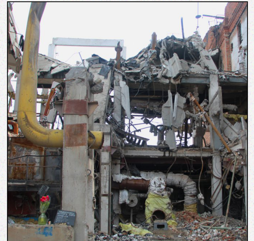
Thermal power station
