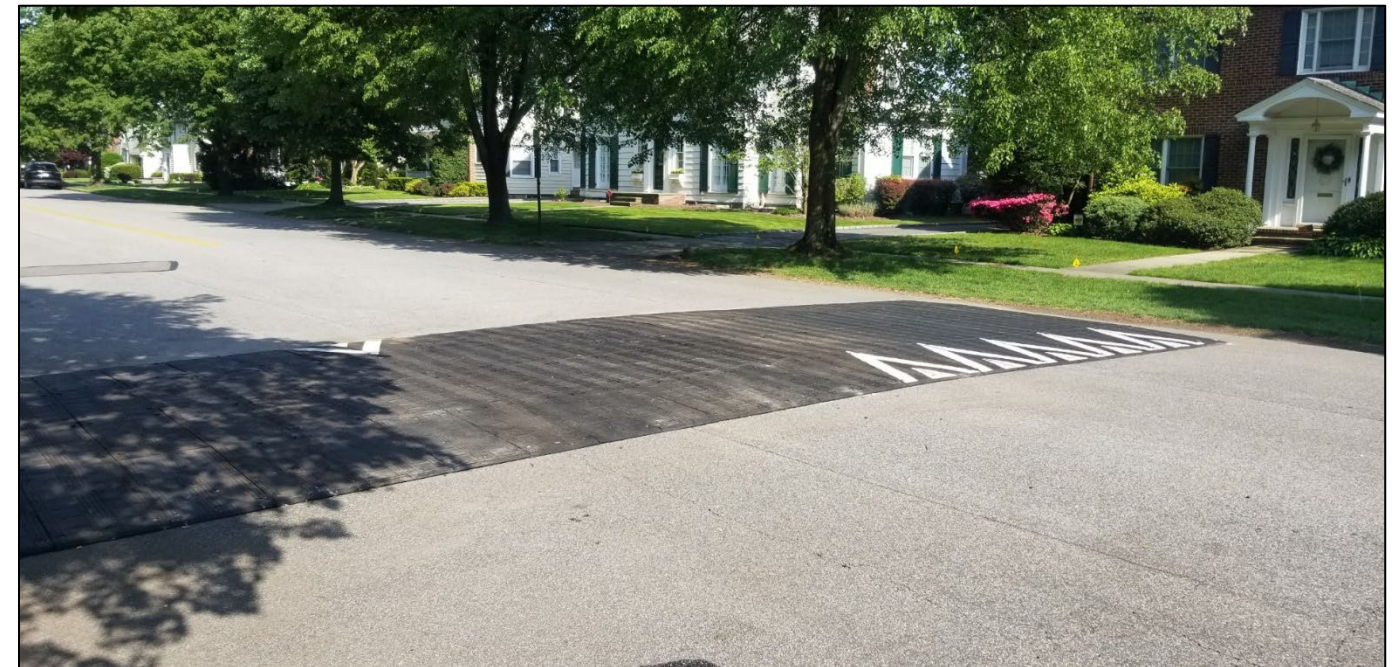
Figure 1: Temporary speed humps have been installed on 4 th Street; this was a recommendation from the prior traffic calming study
