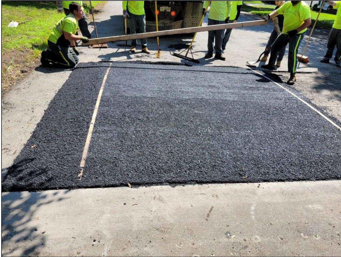
Figure 46: Village staff installing permanent speed humps on 4th St; this was undertaken after the successful temporary speed hump pilot
