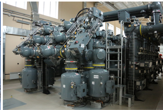
Gas-insulated switchgears 330-750-110 kV
