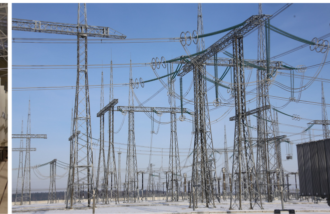
Open switchgear equipment
