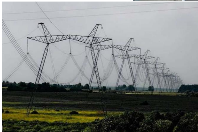
Rivne – Kyiv High Voltage Line 750 kV Zaporizhzhia–Kakhovska Line
