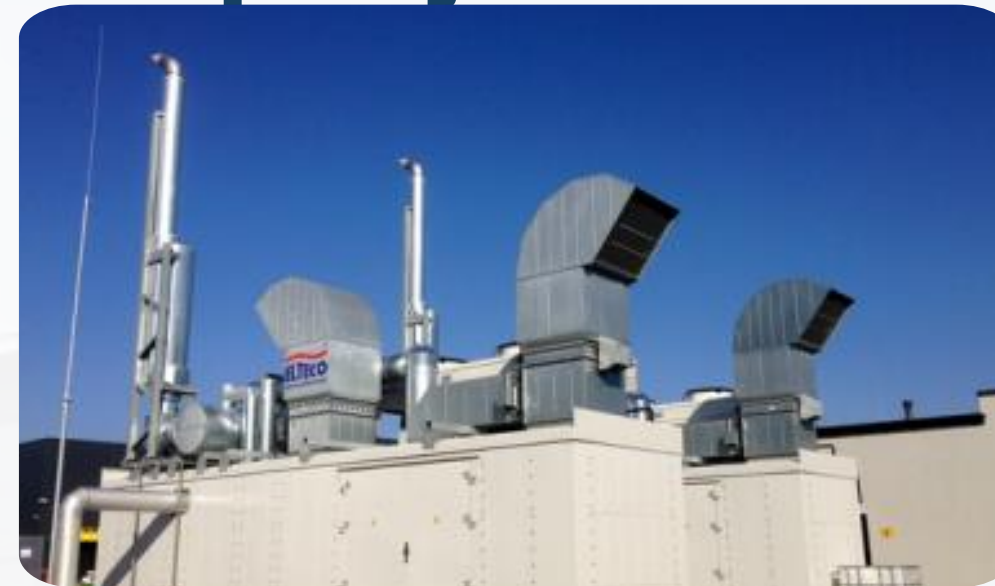
Cogeneration gas piston unit at the Dnipro water treatment plant - 578 894 EUR
