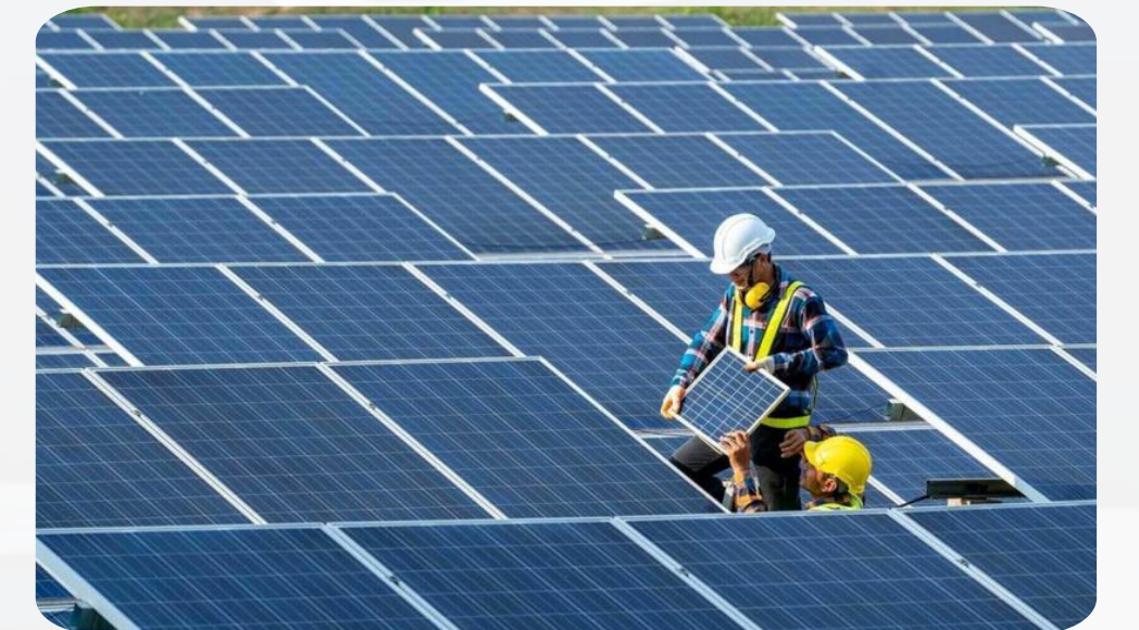
Solar power station at the pumping station - 562 418 EUR
