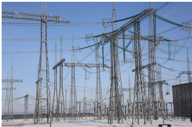
Open switchgear equipment
