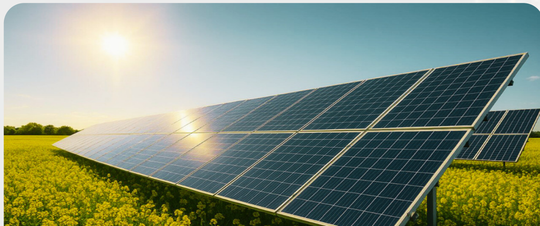
Purchase of a 1 MW modular solar power plant (SPP) at the Vilshanka reserve water intake facility 932 398 EUR
