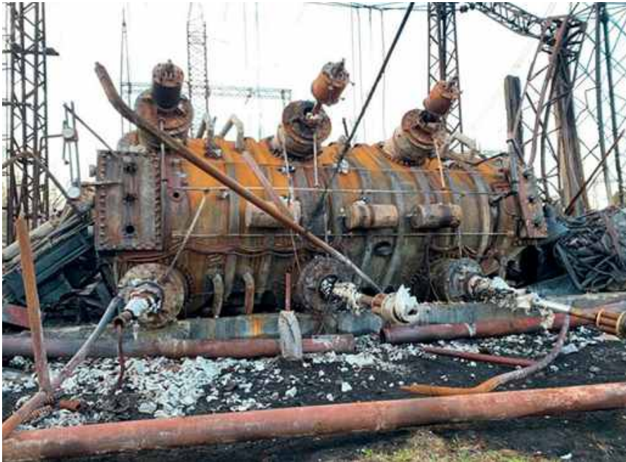
330kV 200MVA Auto Transformer
