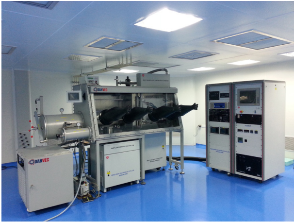
Overall system view placed inside clean room
