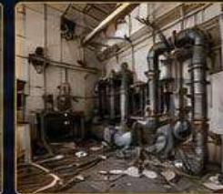
Damaged technical networks
