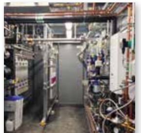
Purification inside the Containers
